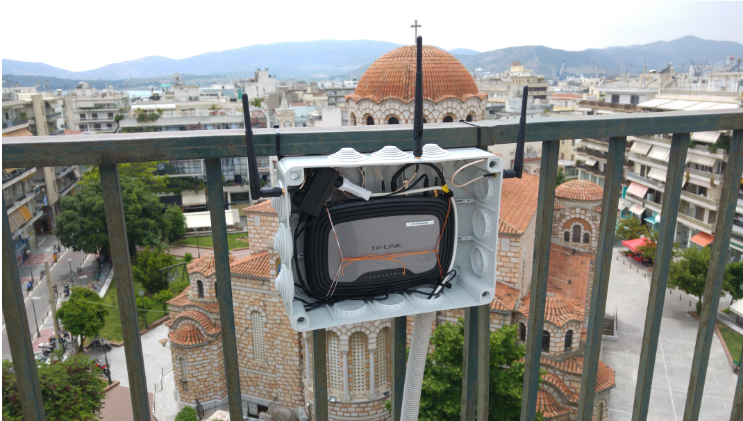
FIGURE 5.3: Monitor DU Device
