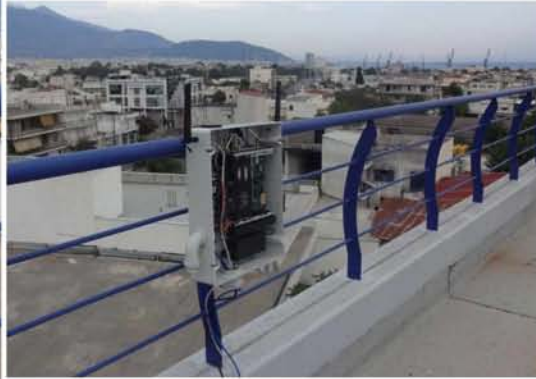
FIGURE 4.4: Outdoor LTE equipment
