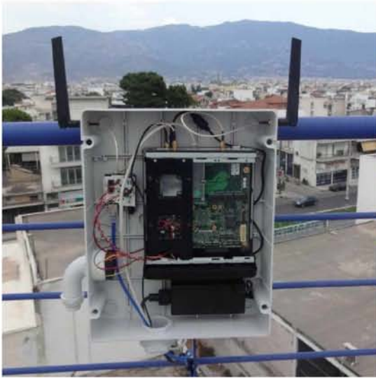
FIGURE 4.3: Outdoor LTE equipment
