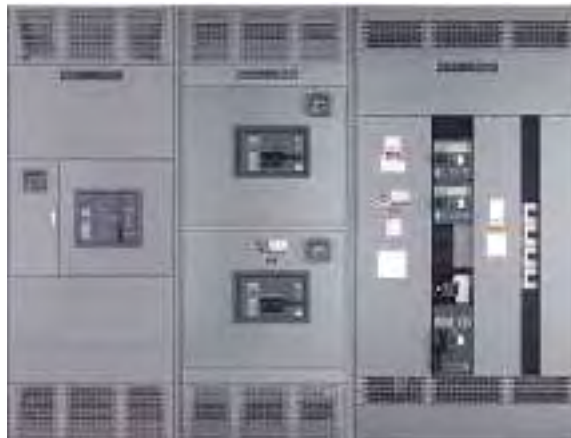
Picture 15 Main Switchboard
