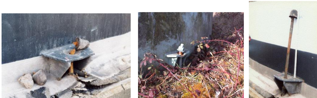
Figure 14: Anchor bolt failure in seismically-loaded tanks.
