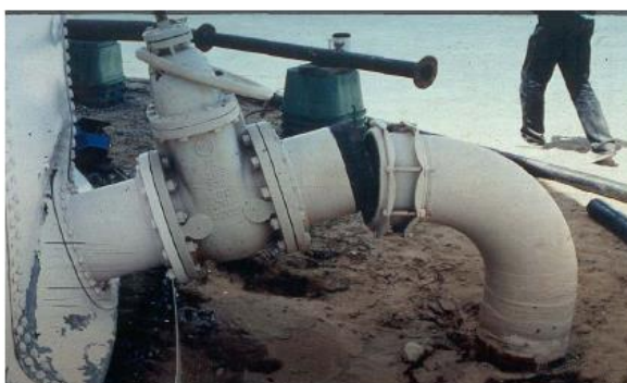
Figure 15: Nozzle (attached piping) failure due to elephant's foot buckling.
