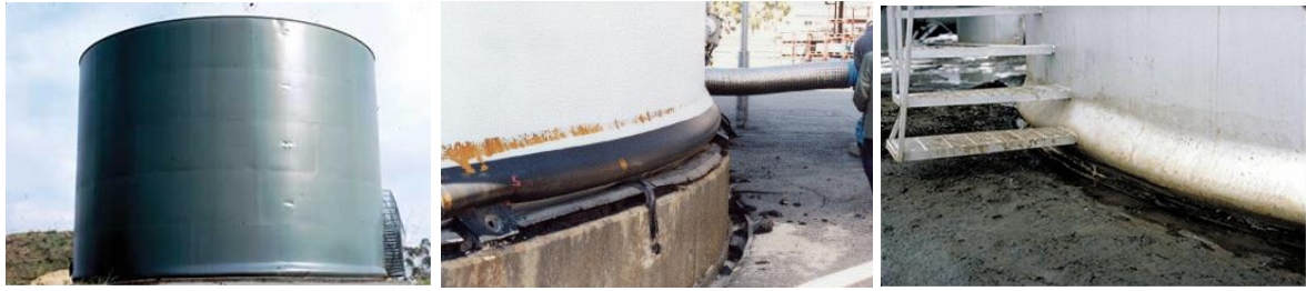
Figure 11: Elephant’s foot buckling caused by strong earthquake action.
