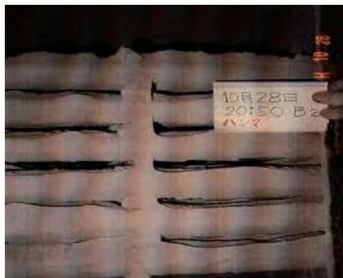
Figure 5.3: Dust deposit in vertical heat exchanger
