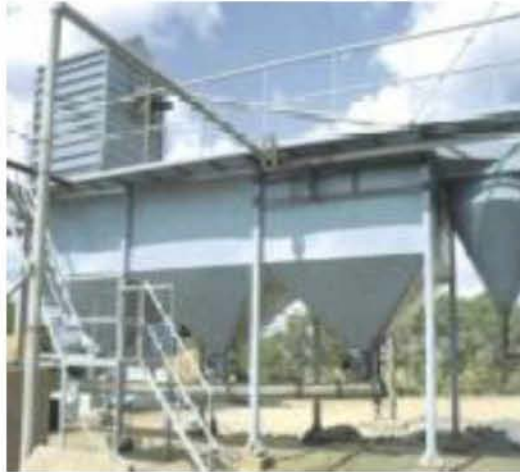
Εικόνα 4.17: Facilities of circulating water treatment
