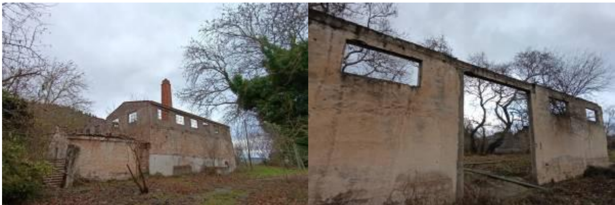
Figure 6.12 Infrastructure of KISSAVOS Tomato Processing Plant
