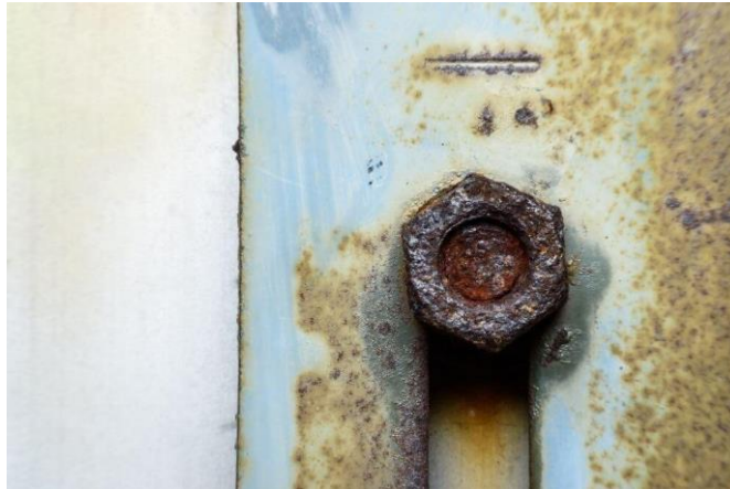
Figure 36: Crevice corrosion thrives at areas around nuts.
