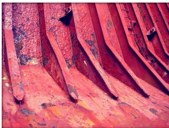
Figure 35: Pitting corrosion at the ship's hopper tanks.
