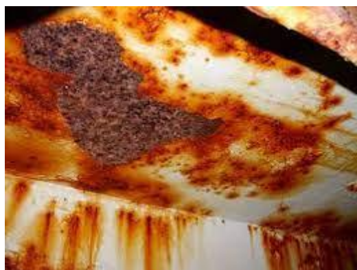
Figure 34: The ship's hull affected by uniform corrosion.
