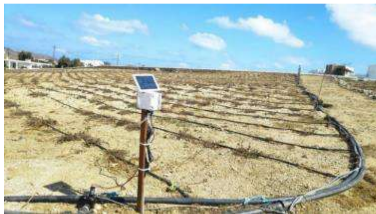
Figure 157: Electrovalve for controlling the water flow
