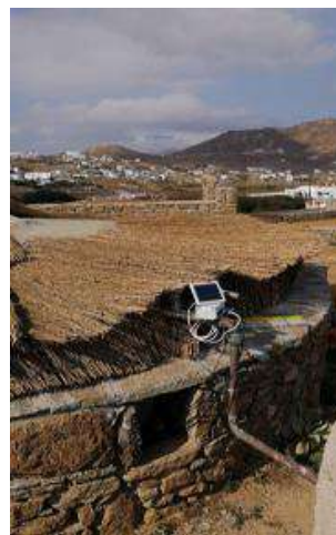
Figure 158: Level sensor installed in one of the tanks.
