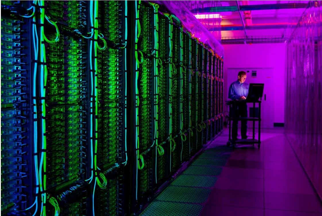
Figure 2.3: A Microsoft cloud computing center in Quincy. This is what a modern data storage facility looks like where millions of gigabytes are stored. Wash. Credit...Richard Duvall. Picture taken from https://www.nytimes.com/2017/01/23/insider/where-does-cloud-storage-really-reside-and-is-it-secure.html
