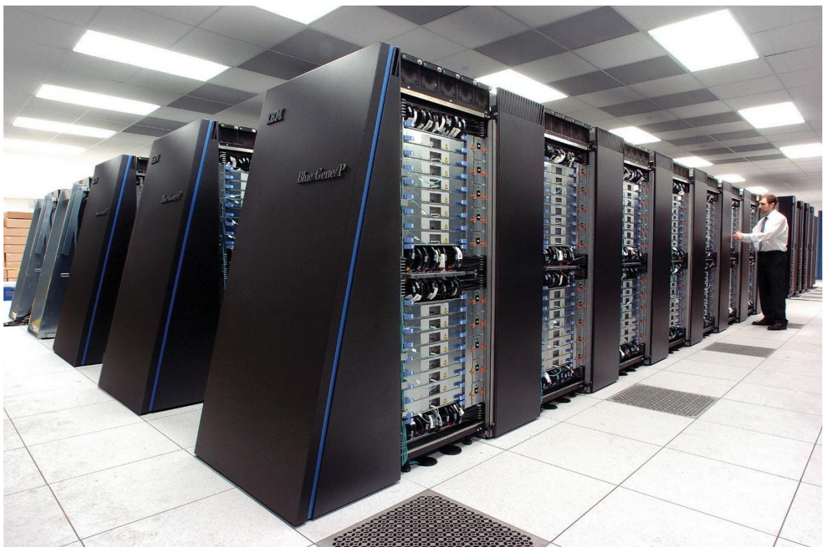
Figure 2.2: The IBM Blue Gene/P supercomputer installation at the Argonne Leadership Angela Yang Computing Facility located in the Argonne National Laboratory, in Lemont, Illinois, USA. All modern supercomputers utilize the power of clustered machines. Taken from https://commons.wikimedia.org/wiki/File:IBM_Blue_Gene_P_supercomputer.jpg
