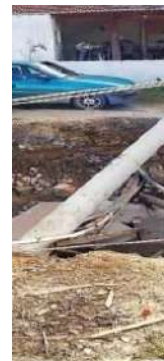
Picture 10: The fallen electricity pylon
