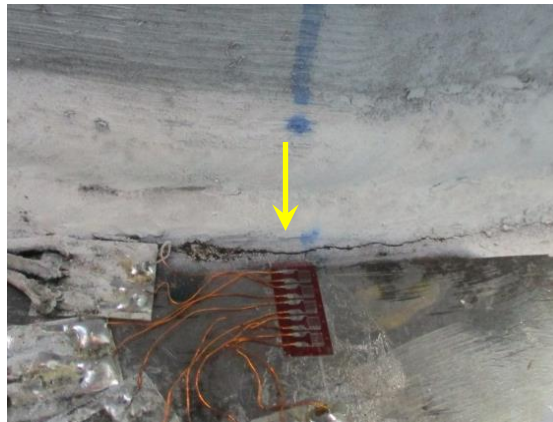
first crack detection ( \approx 3,000 cy)
