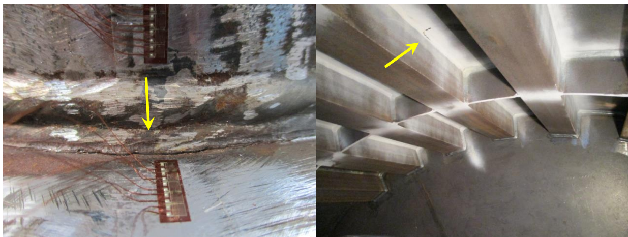
Figure 14: Crack at crown position (left), Crack at the “inner” skin side – stiffener (right)
