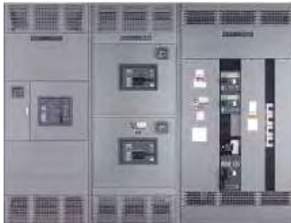
Picture 15 Main Switchboard
