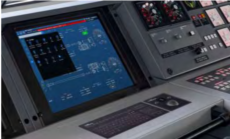
Picture 16 Alarm Monitoring and Control System (AMCS)
