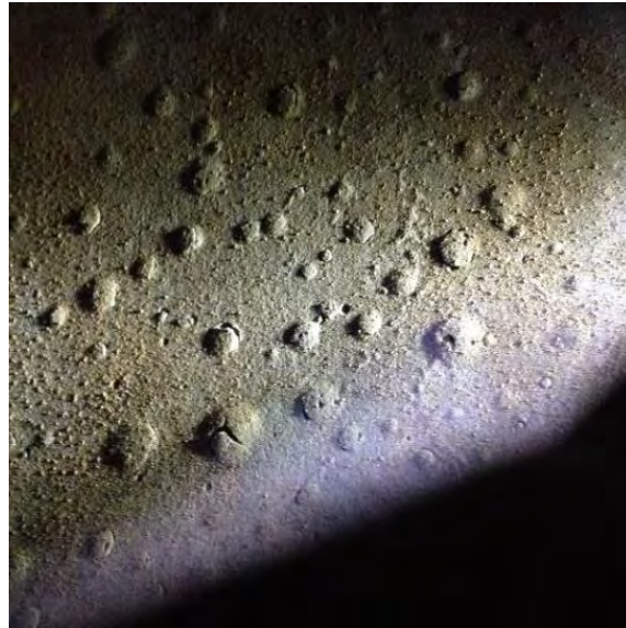
Figure 7. Blistering in internal surface
