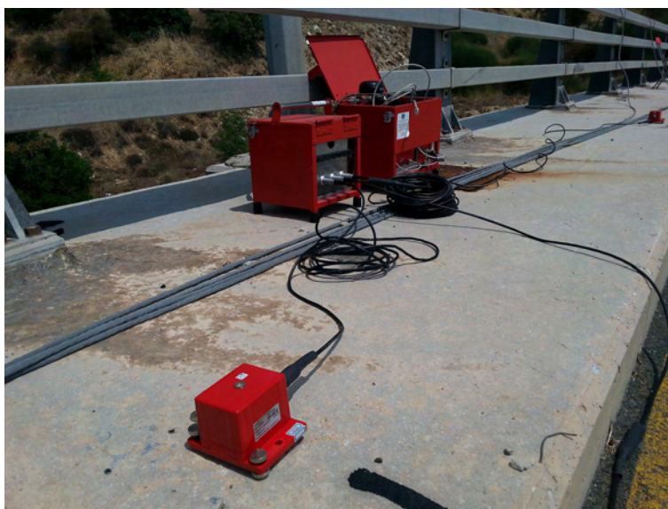
Figure 4.10: Uniaxial accelerometer, junction box, and unit including recorder, battery pack and GPS module
