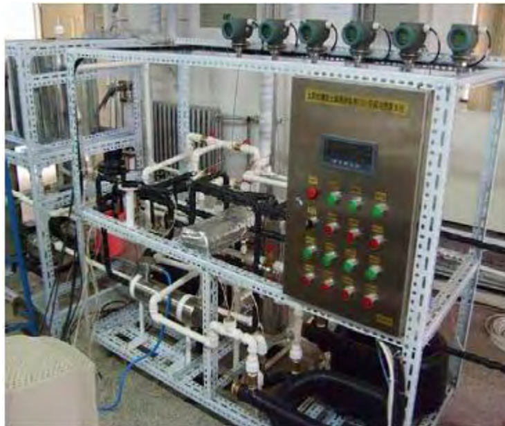
Figure 18. A photograph of ground source CO2 air conditioning and heat pump system [18]
