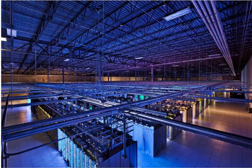
Figure 11: A central cooling plant in Google's Douglas County, Georgia, data center.
