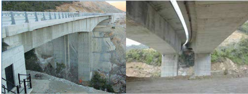
(a) (b) Figure 1.2: (a) Longitudinal Section of G9 Polymylos Bridge , (b) Transverse Section of G9 Polymylos Bridge .
