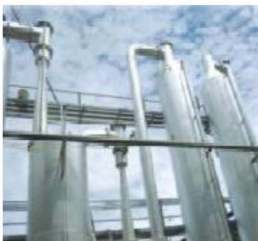
Εικόνα 4.15: Device of cleaning and cooling system
