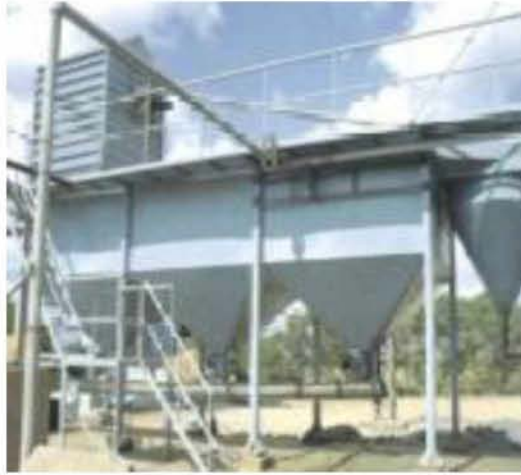
Εικόνα 4.17: Facilities of circulating water treatment
