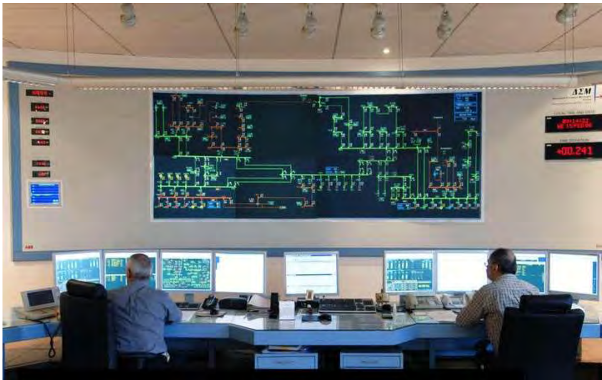
Figure 3. The National Energy Control Centre of Cyprus
