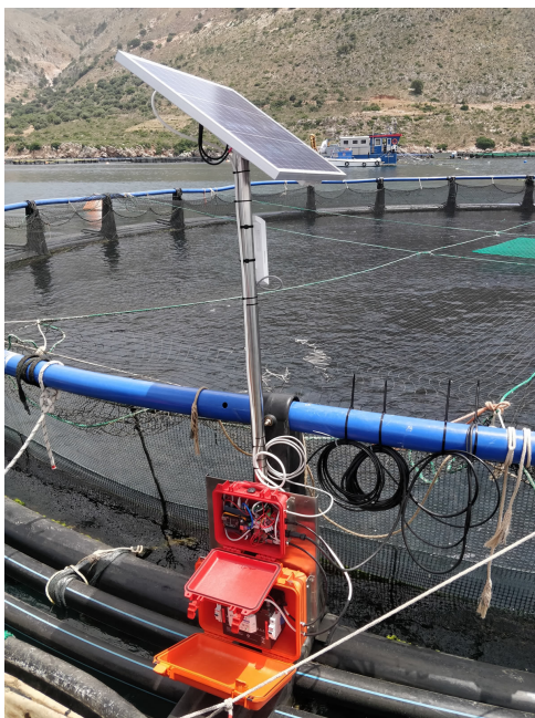
(A) Overwater System w/ Solar Panel
