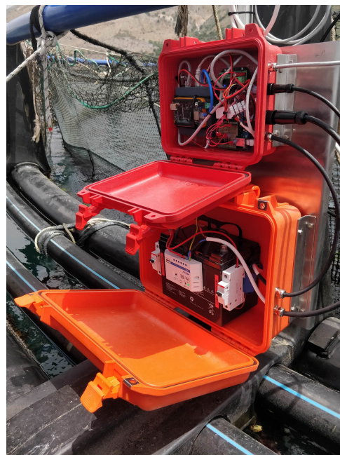
(B) Utilized Electronics and Battery
