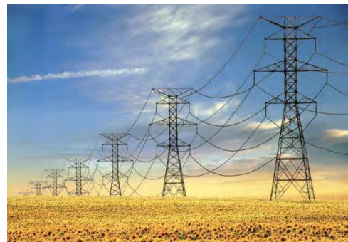
Figure 3: A transmission line
