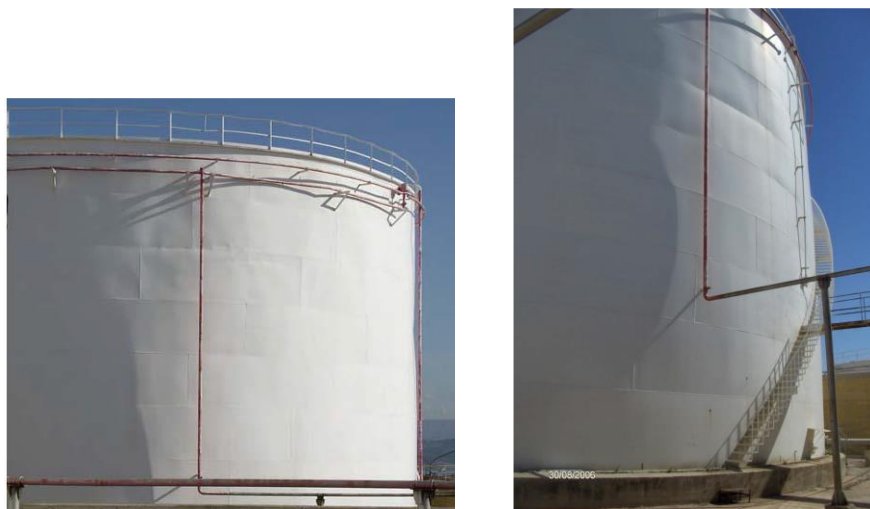
Figure 22: The tank used for the measurements.
