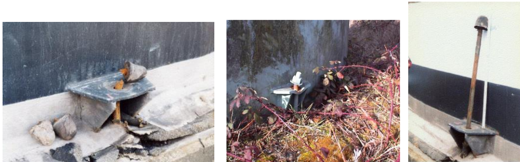
Figure 14: Anchor bolt failure in seismically-loaded tanks.
