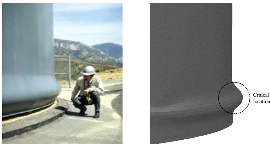
Figure 17: Elephant's foot buckling in liquid storage tanks (a) existing tank (Malhotra 2000), (b) buckling shape from present finite element analysis.
