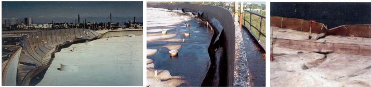
Figure 16: Failure of floating roof.
