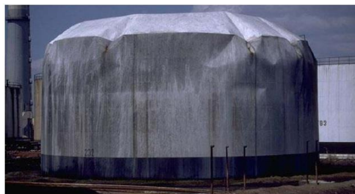
Figure 12: Tank roof damage due to sloshing; Kocaeli, Turkey earthquake 1999.
