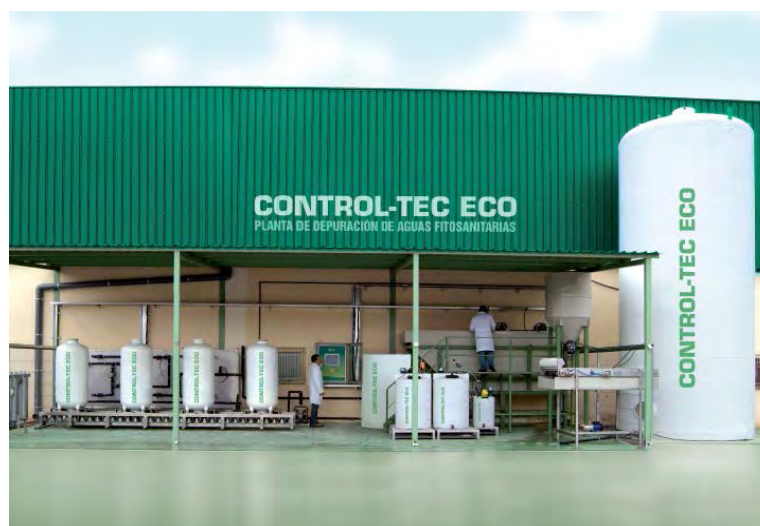
Photograph 1.1. The Control-Tec Eco® system used for the treatment of effluents from fruit packaging plants
