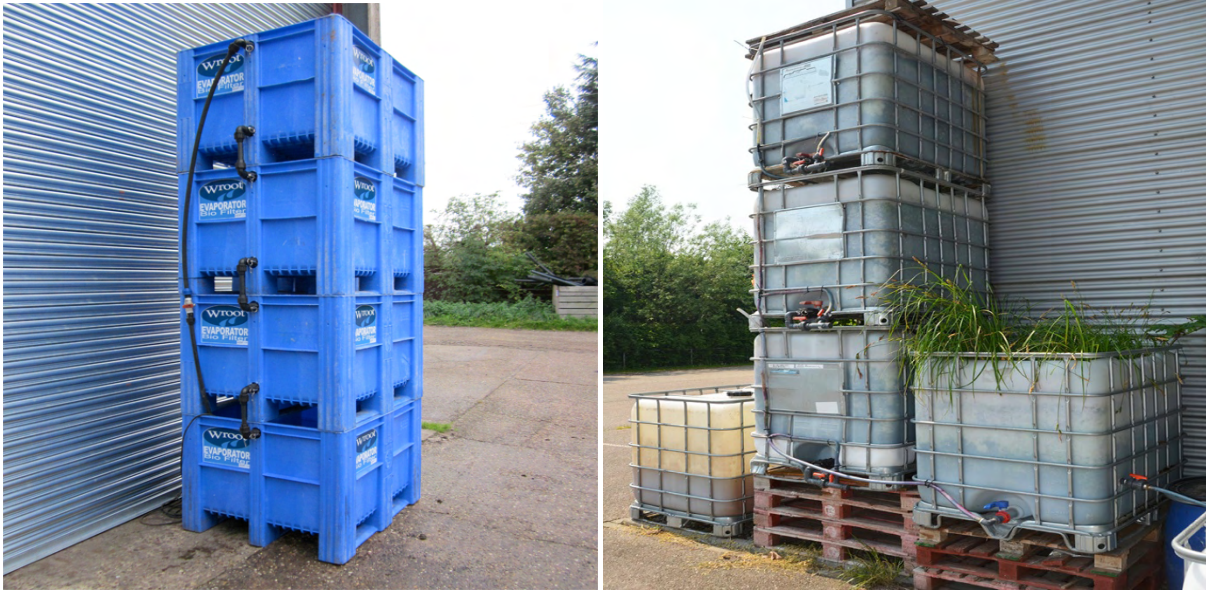
Photograph 1.2. Typical biofilters installed in Belgium (source: http://biobeds.net/en/modified-biobed-systems/ , http://wrootwater.com/index.php/water-treatment-2/bio-beds-bio-filters/ )
