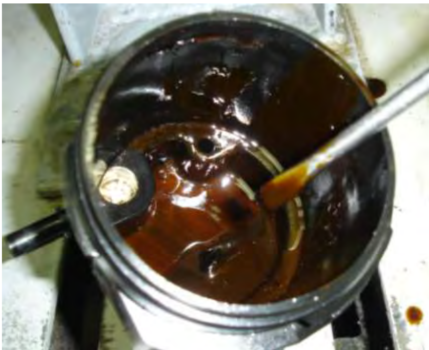
Figure 8.1. Fuel filter box. Significant quantity of brown dense slurry was found at the bottom of the box.
