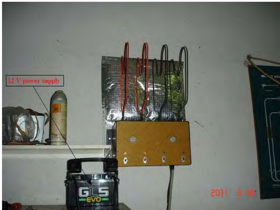
Figure 3.4: The 4-resistance device with the battery. 2/4 resistances are operating.
