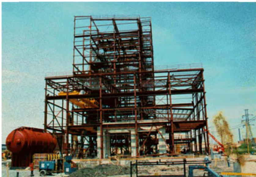
Niagara Cogeneration Project, Niagara Falls, New York was designed by Southern Electric International, Inc.
