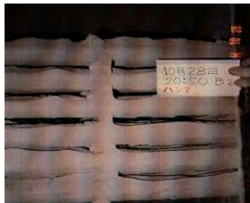
Figure 5.3: Dust deposit in vertical heat exchanger
