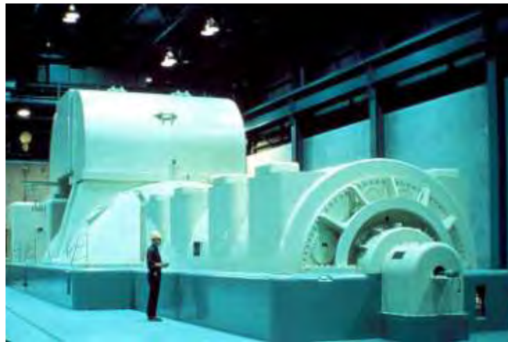
Figure 5.4: Modern steam-turbine generator
