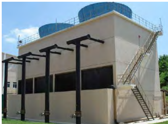
Figure 5.5: Water cooling station
