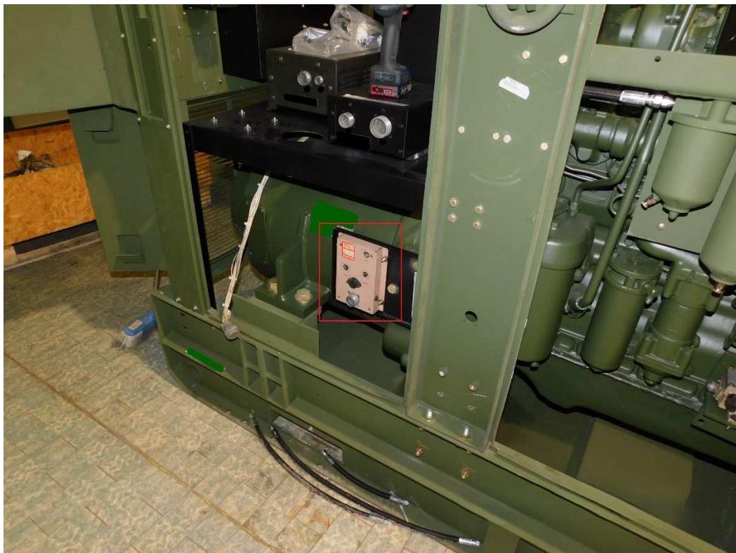
Figure 3.23. Generator ECU and regulator openings for coverage
