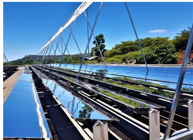
Figure 6: Linear Fresnel reflectors
