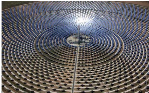
Figure 3: Concentrating solar tower
