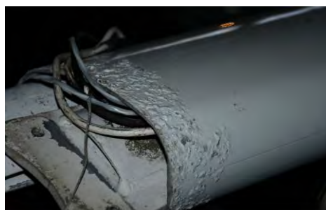
Figure 3. 5 Galvanic Corrosion on a mast that appears as bubbles.
