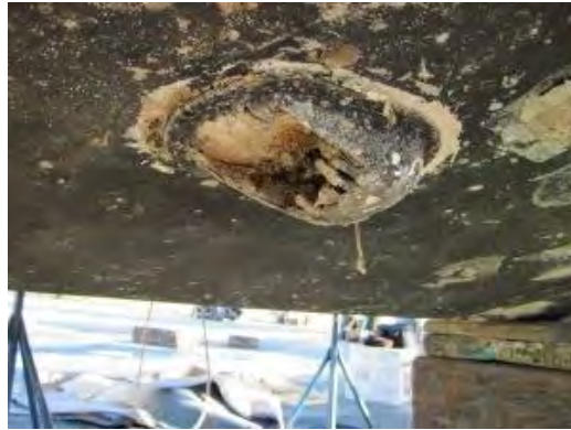
Figure 3. 31 Bronze intake strainer destroyed from galvanic corrosion.
