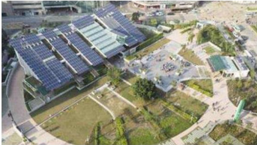
Figure 7.3: Solar PV panels installed onsite [114].
