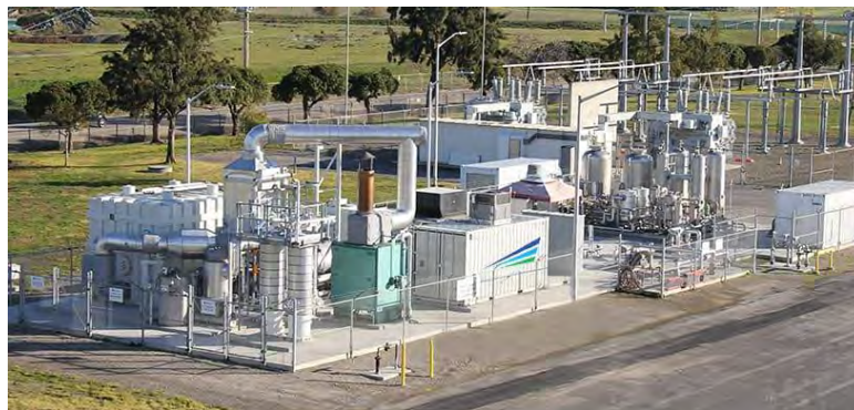
Figure 14 : Fuel cell stationary power facility [14].
