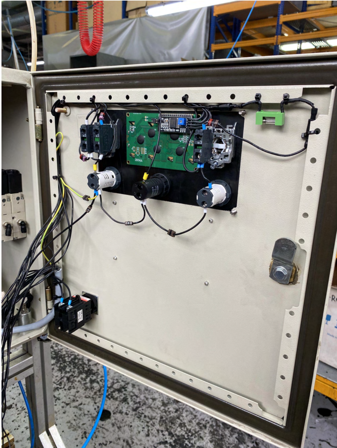
Figure 4.2: The control panel (rear view)
