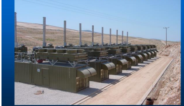
Biogas plant in Ano Liossia - Cogeneration unit
