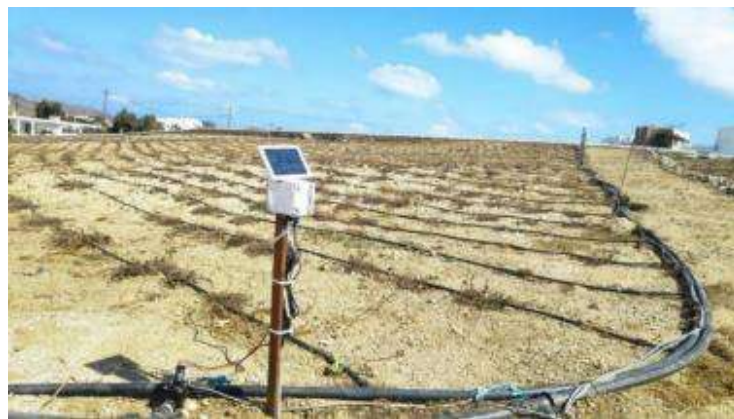
Figure 157: Electrovalve for controlling the water flow
